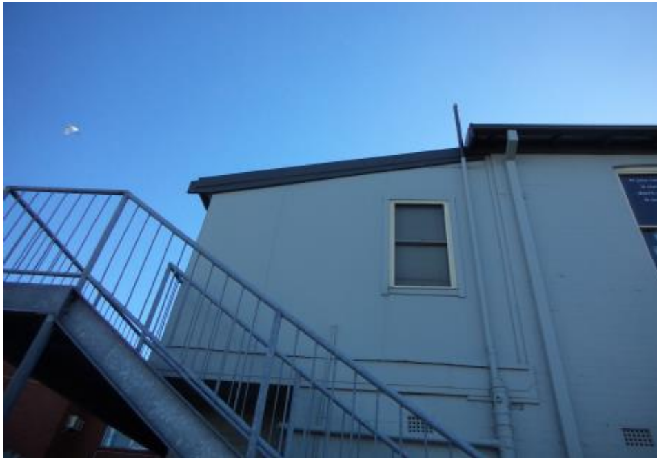
Photo 15 - 125, External, presumed asbestos cement cladding to level 1 rear extension.
