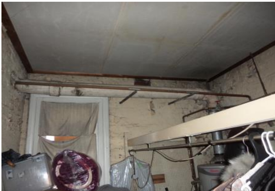
Photo 8 - 123, Ground floor, presumed asbestos flue, asbestos ceiling lining above Rheem HWU.
