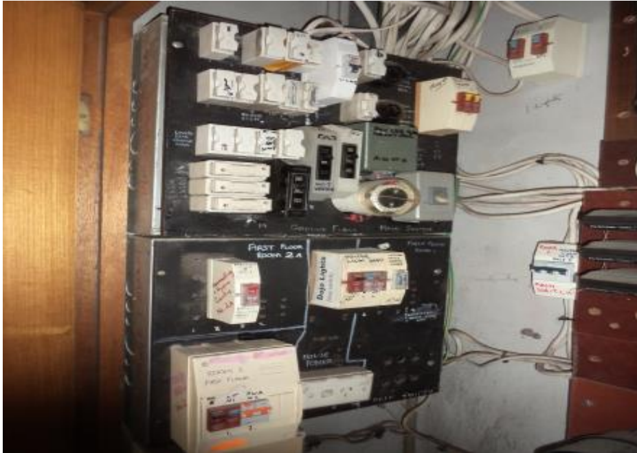
Photo 3 - 117-119 Internal, ground floor, asbestos backing boards.
