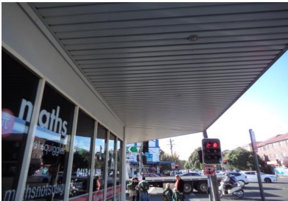
Photo 16 - 125, External, presumed asbestos cement panels over windows.
