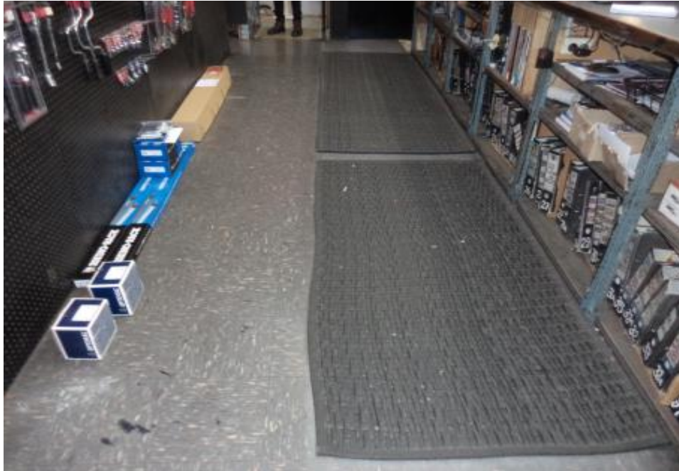
Photo 5 - 117-119 Internal, ground floor, presumed asbestos floor tiles.
