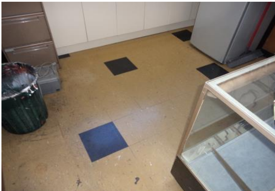
Photo 6 - 117-119 Internal, ground floor, presumed asbestos floor tiles.
