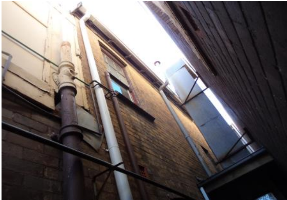
Photo 19 - 121-123, External, flaking paint systems.
