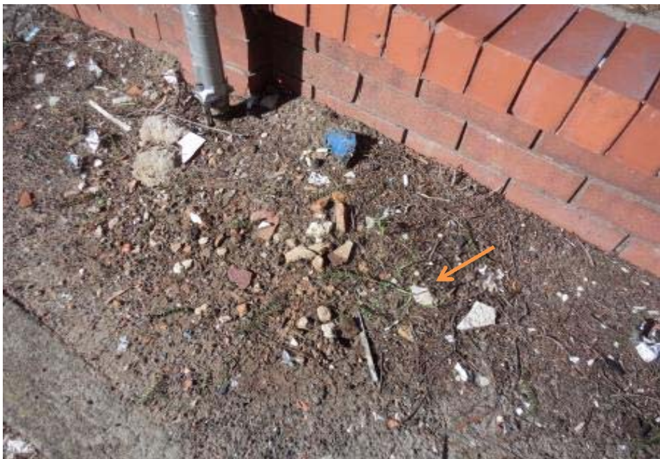
Photo 18 - Externals, Auto-one car park, flower bed, presumed asbestos cement fragments.
