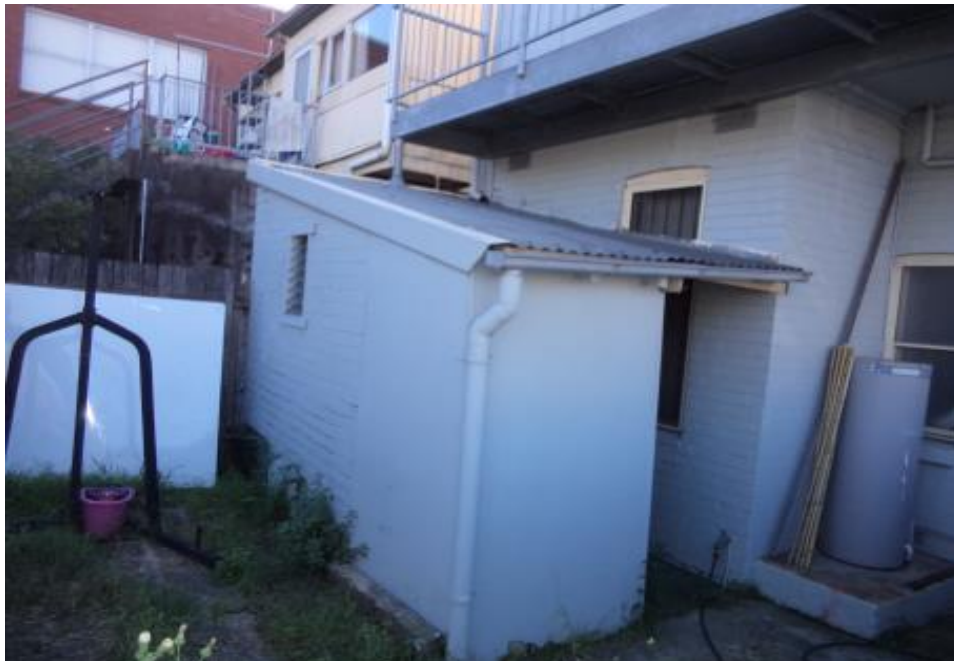
Photo 14 - 125, External, presumed asbestos cement cladding to utility room.
