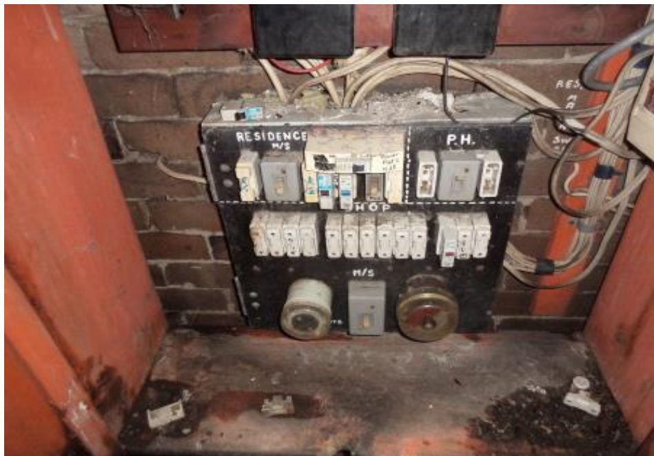
Photo 10 - 123 External, ground floor, presumed asbestos backing board.
