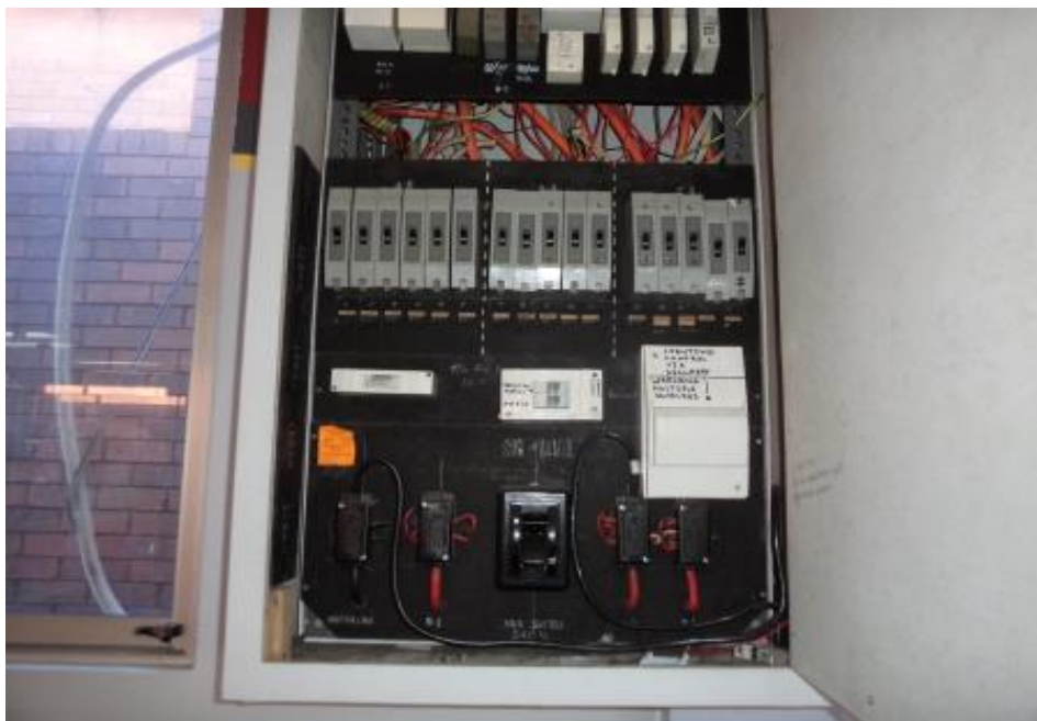
Photo 2 - 113-115 Internal, level 1, asbestos backing boards and presumed cement linings.
